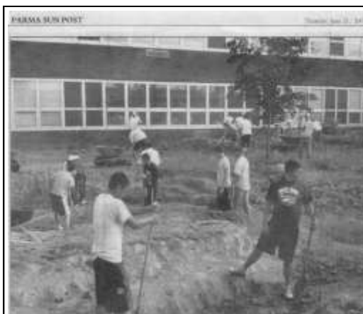
And so the project continues. Major digging went on in May and there have been great strides ever since. We wish to publicly thank Marco's Pizza, PJay's Pizza and Marc's Inc. for donating pizza and drinks for our hard workers!
